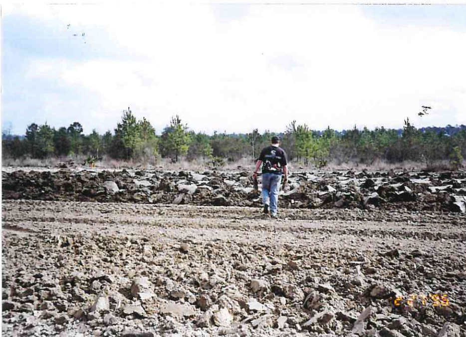
15.Southeast arm at station 114+00 spreading out excavated fill to start the drying process.
