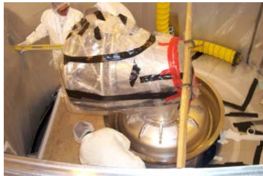
Cathode inside vacuum vessel
