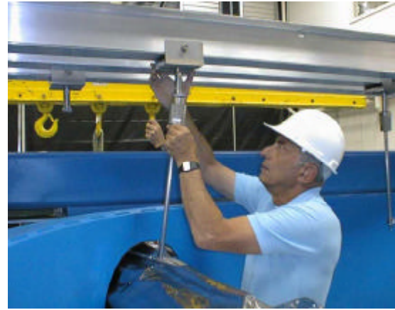
Figure 22. Trolley Linkage Connected to Support Tube.
