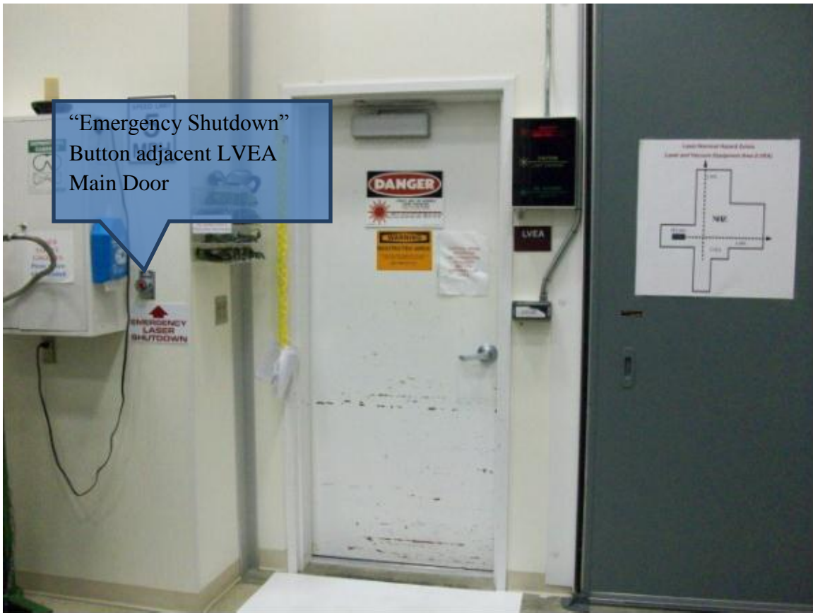
Figure 10: The location of “Emergency Shutdown” button adjacent the LVEA main entrance.
